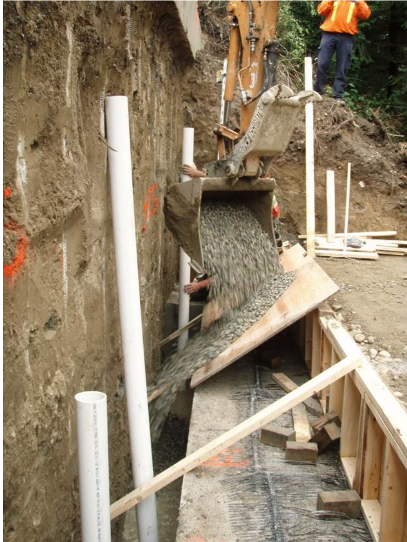
Figure 11. Placing the leachate collection gravel with the vertical collection pipes. CDF wall placed.
